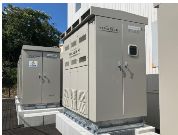
Large-capacity Li-ion storage batteries
