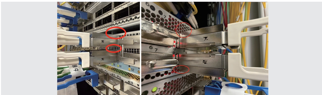
Figure 2: Examples of 400ZR Cooling Mechanism
